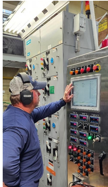
S-8 Engine Control Panel Upgrades
